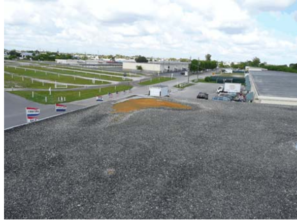
Figure 7: Typical scour pattern (Roof No. 4).
