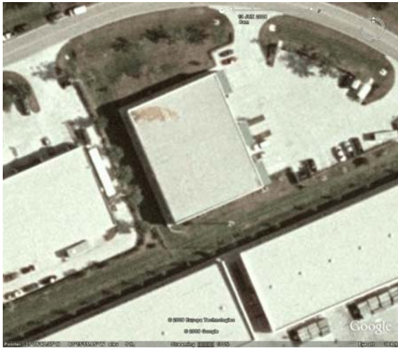
Figure 8: Typical scour pattern (Roof No. 2). Photo courtesy Google Earth.
