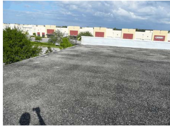
Figure 4: Discontinuous parapet on Roof No. 2.
