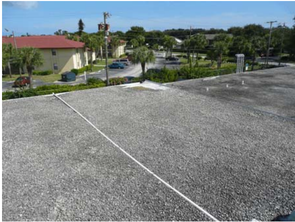
Figure 6: Typical minor scour (Roof No. 16).
