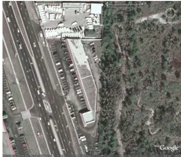
Figure 9: Roof No. 13 exhibited aggregate loss. Roof had no parapet on the side facing Exposure C. Aggregate loss was from the northern half of this roof. Photo courtesy Google Earth.
